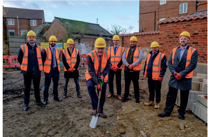
Breaking the ground at the Swinegate development. Pictured are, left to right, Matthew Jones (Lindum Group Framework Manager), Steve Angus (Lindum Commercial Director), Richard Wyles (SKDC Deputy Chief Executive), Cllr Phil Dilks (SKDC Cabinet Member), Cllr Matthew Bailey (SKDC Ward Member), Suniel Pillai (SKDC New Build Project Officer), John Ginnelly (Contract Manager), Owen Cheshire (Scape).
