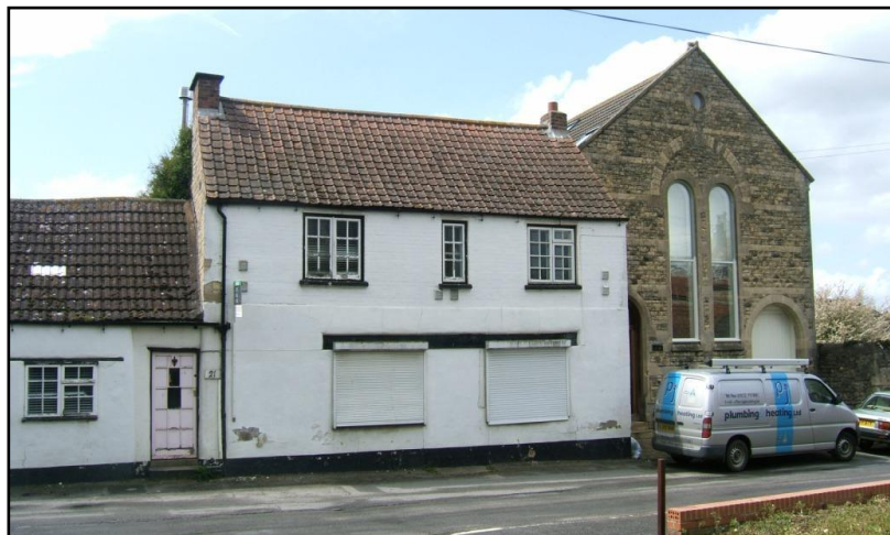
Fig. 9 21 Church Street is in a deteriorating condition and would benefit from maintenance works to improve its appearance in the conservation area.
