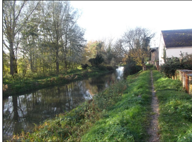
Public footpath alongside the River Welland to the south of Stamford Road is in need of maintenance to allow improved access and safety for users.
