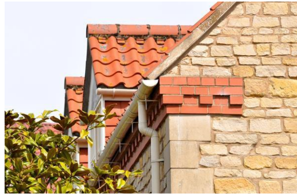
Gabled dormers and red brick oversailing courses with coursed limestone rubble walling .
