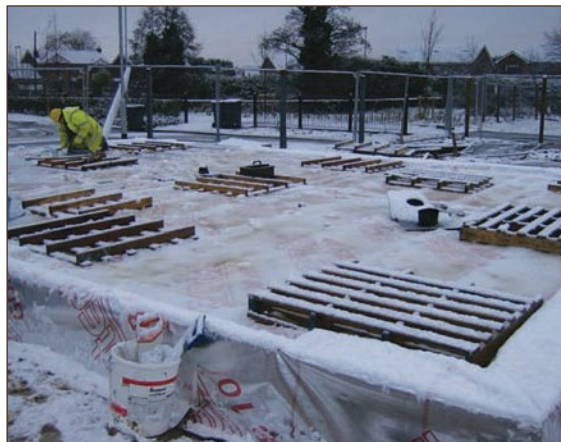
Figure A4.84 Taped joints are difficult to construct in adverse weather. Also difficult to inspect if covered with snow (courtesy Smith Grant)
