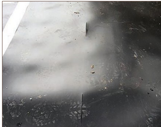
Figure A4.58 Damage caused to gas membrane by follow-on trade who cut/shaped the dry lining board directly on the unprotected installed gas membrane (courtesy NHBC)
