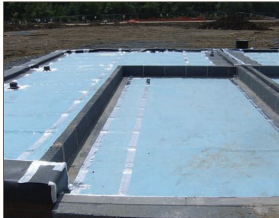
Figure A4.10 Almost complete coverage available for inspection, minimal jointing, service entries suitable distance from walls, light traffic (courtesy Smith Grant)
