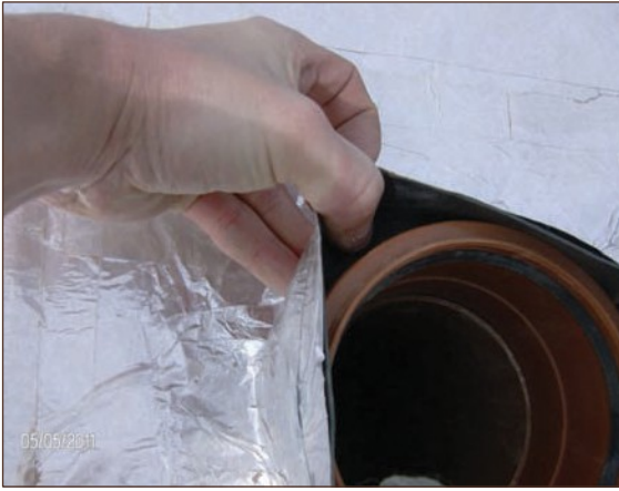
Figure A4.73 No bead of double sided butyl tape provided between interfaces of ID top hat and OD service pipe: cannot be compressed enough to form seal (courtesy Smith Grant)
