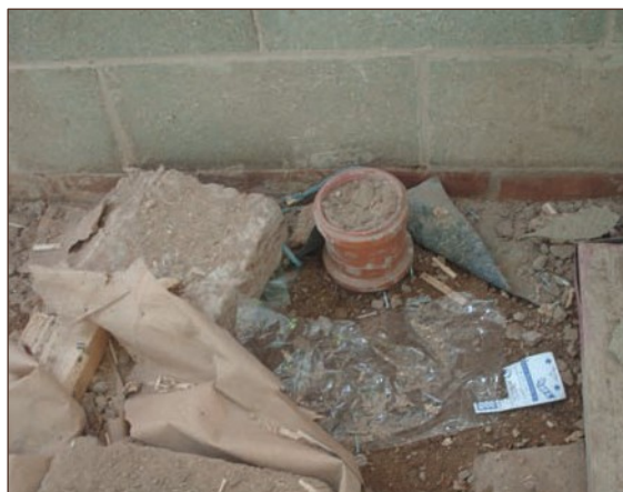
Figure A4.48 Loose nails and over construction debris likely to be left in place beneath gas membrane – poor preparation of gas membrane prior to sealing service penetration (courtesy Card Geotechnics Limited)
