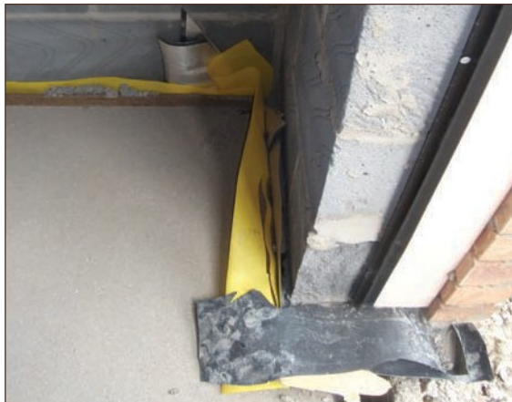
Figure A4.70 Inadequate corner detailing. The use of preformed proprietary products would have avoided such bad practice (courtesy NHBC)
